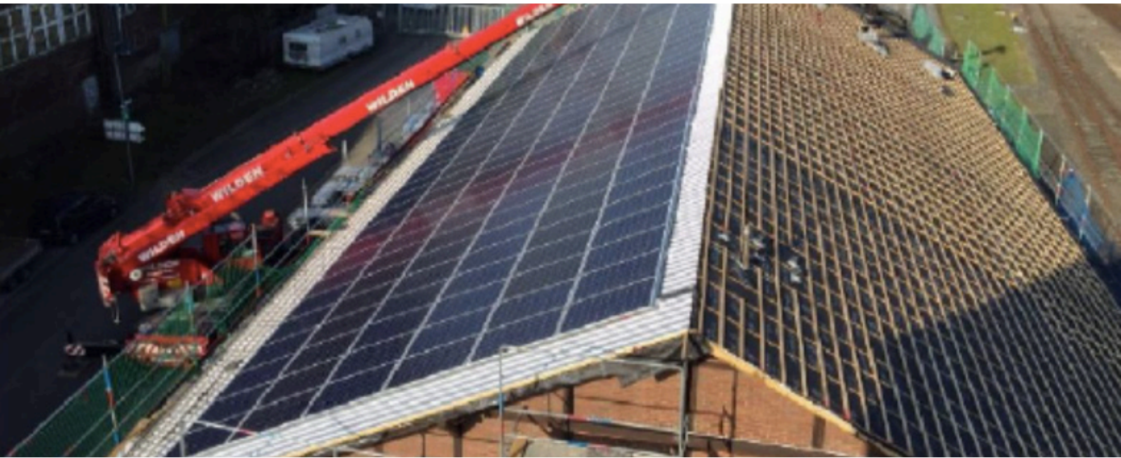
120 kWp Rooftop Mettman Bahnhof, Germany
